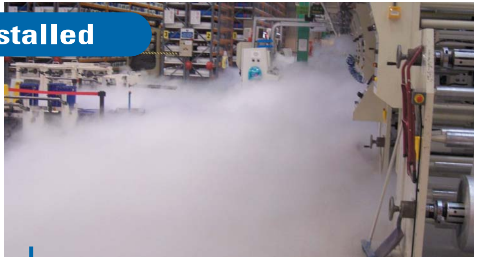
The CO2 system in action.
